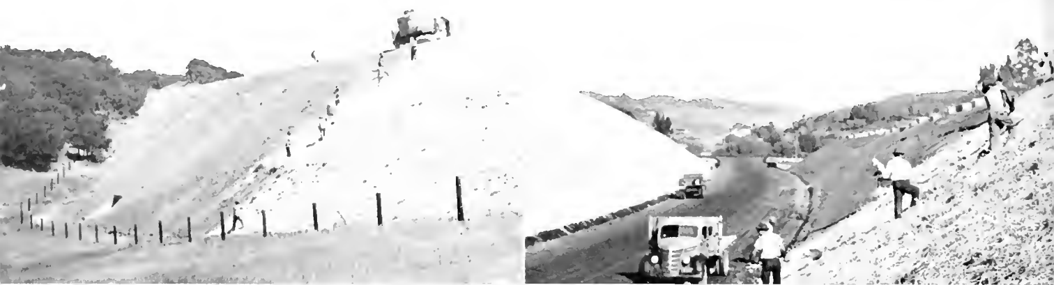
Fill slope treatment. Half of seed is sowed before straw is applied
